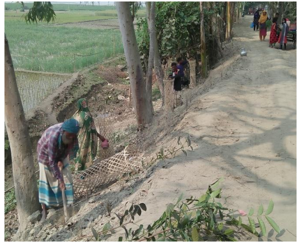
Grass & tree planting to protect the road from flood at Kulkandi, Islampur.
